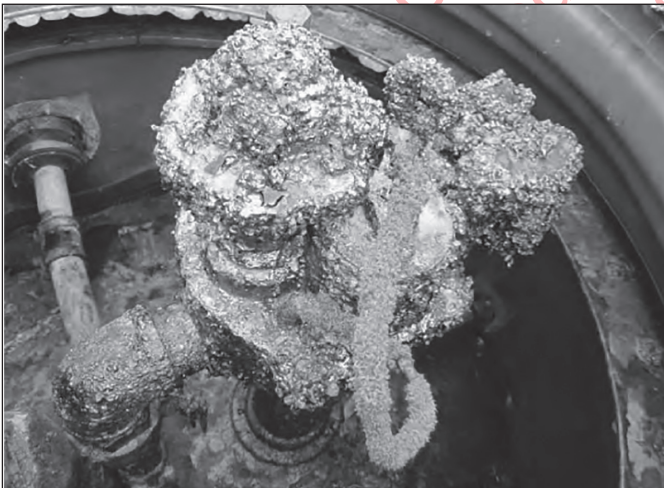
FIGURE 7-1. Corrosion may form a thick, rough layer on metallic components located above tanks containing ethanol-blended gasoline. This type of corrosion is caused by microbes that feed on ethanol and produce acid that is responsible for the corrosion.
