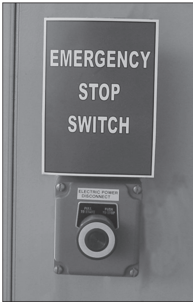
FIGURE 5-1. The emergency stop switch immediately cuts off power to all fuel dispensing equipment. All employees and service personnel should know where this switch is located and under what circumstances to use it.
