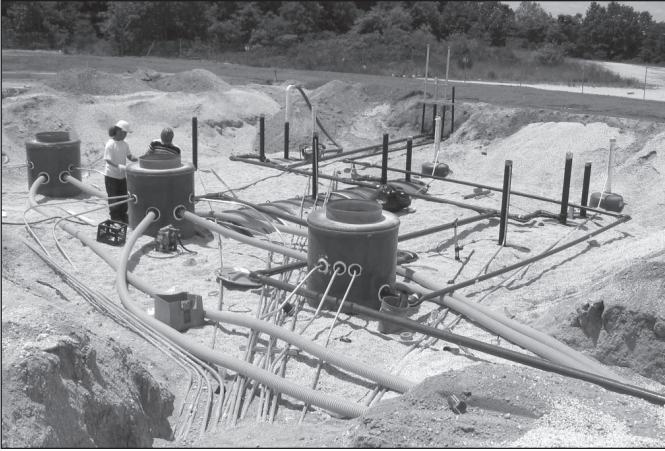
FIGURE 1-2. Once tanks are installed and backfilled, many different types of equipment must be connected to the tank top. Ongoing inspection and maintenance of this equipment is essential to ensure the safe and efficient operation of the storage system.
