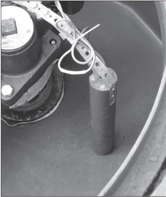
FIGURE 7-5. Verify that sump sensors are mounted vertically and in contact with the bottom of the sump. Test the operation of the sensor to verify that it is functional.
