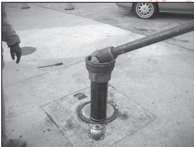
FIGURE 7-3. To avoid damage when removing or reinstalling the ball float, use an extractor tool recommended by the ball float manufacturer.
