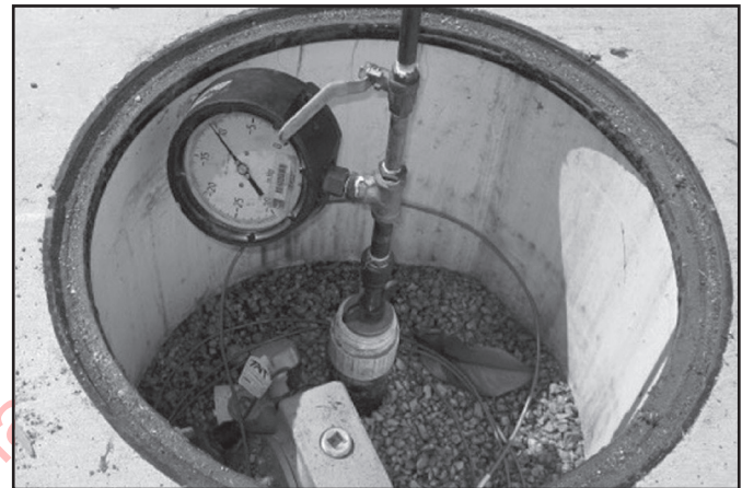
FIGURE 4-3. The vacuum gauge and control valve used for tank interstitial testing.
