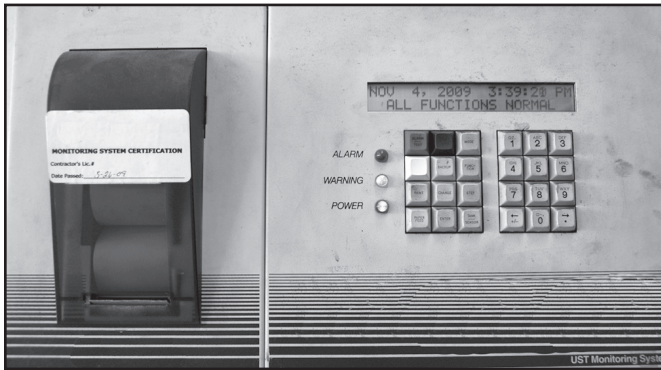
FIGURE 8-1. The indicator lights and the LCD display on the monitoring console show the status of the UST system.
