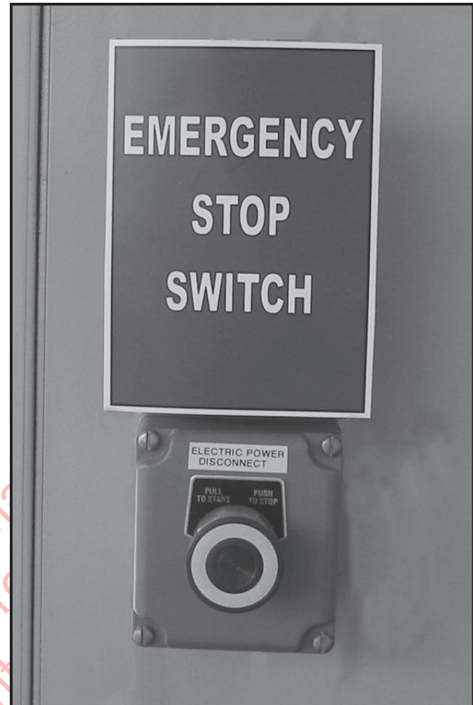
FIGURE 11-1. The E-stop should be clearly labeled and located where it is easily accessible.
